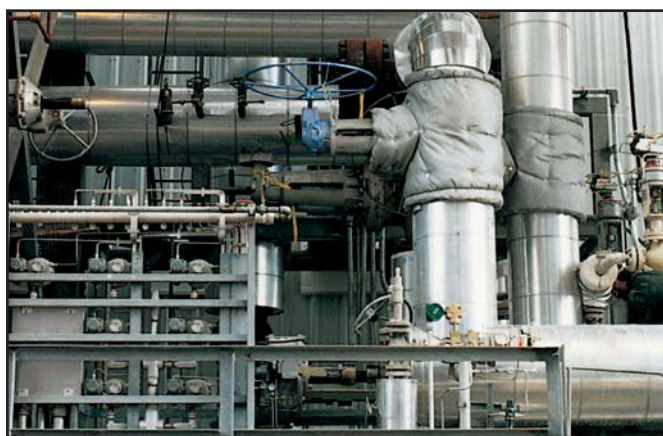
Pressure seal valve in a cogenation power plant.
